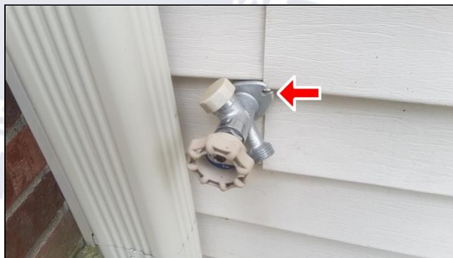
1.7 Item 1(Picture) Front hose faucet
