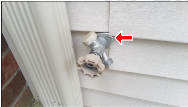
1.7 Item 1(Picture) Front hose faucet
